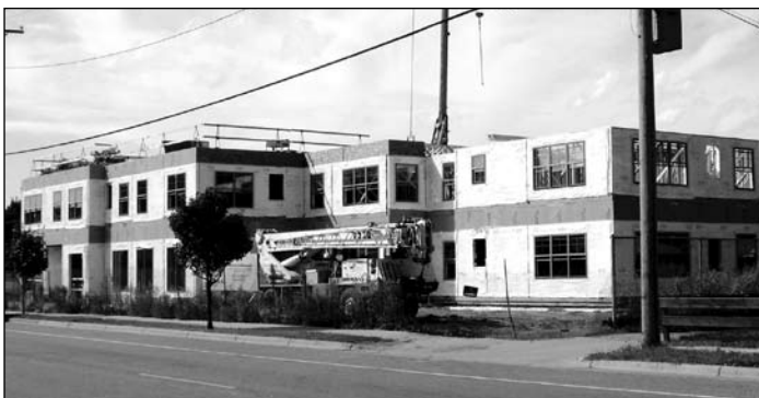
Construction on The Waters of Minnehaha, an assisted-living facility at 3717 23rd Ave. S., rose quickly above the ground this summer. At the end of August, this façade faced 38th St.
