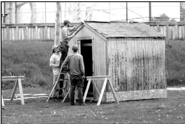
Steve Nichols, Brian VanHout, and Spencer Anderson reconstructed a donated shed at Southside Star Community Garden (32nd Ave. S. and E. 41st St.).
